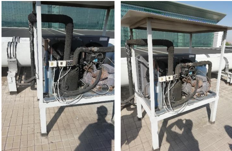
Current condensing unit to be removed, maintain the base without a roof for the new one
