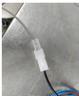
Connection Gray Cable #12 and Black Cable #1
